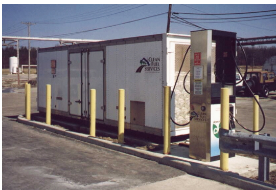
Figure 1. On-Site CNG Fueling Facility
