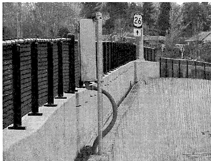
Figure 7.2: Wall 14 control panel
