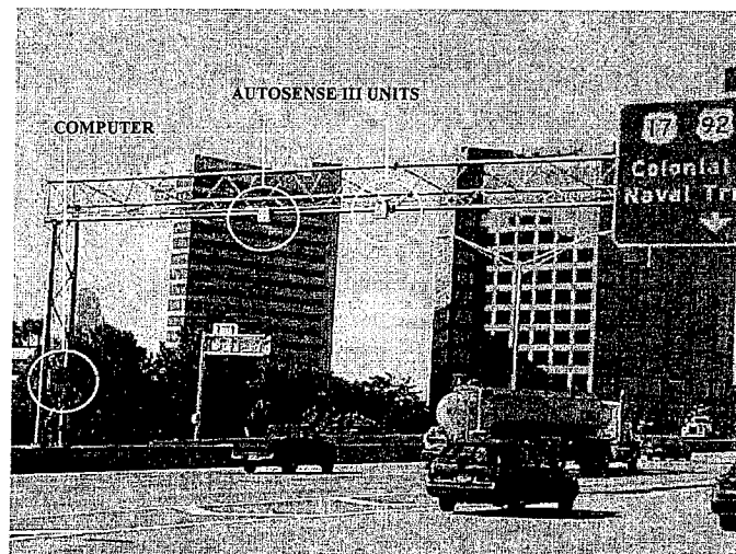
Figure 1: Autosense III Installation on I-4. Two Autosense III Units Installed on the Interstate 4 Sign Structure at the Lake Ivanhoe Interchange on Westbound I-4
