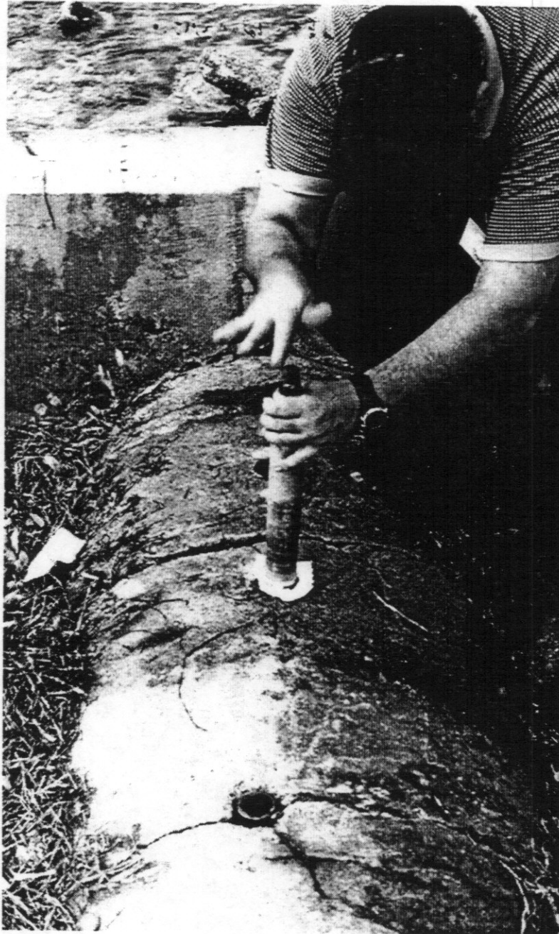
Figure 30. Site No. 7. End of San Jose Street. Low Tide. Core extraction. Evidence of pipe distress.
