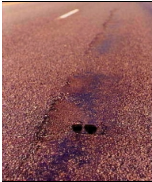
Figure 3.14: Close-up Image of I-84 Stripping, 1997
