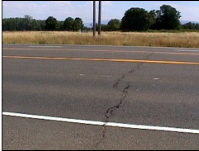
Figure 4.23: Transverse Crack on ORE 99 at MP 111.5 SB
