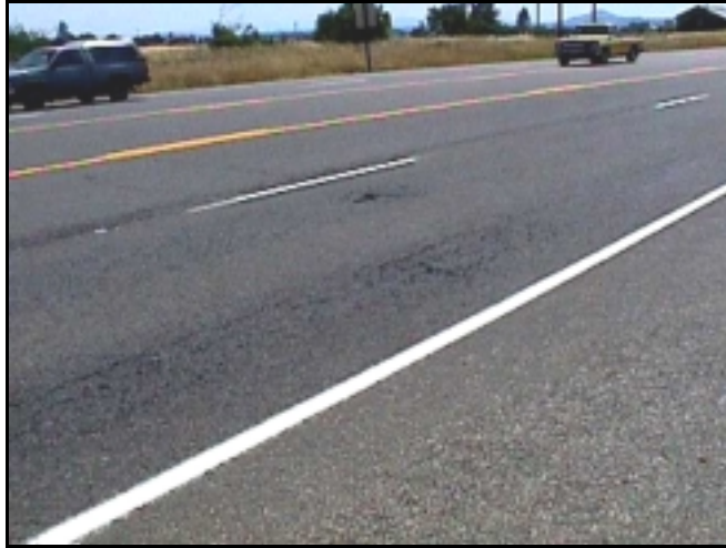
Figure 4.26: Raveling on ORE 99 at MP 114.1 SB
