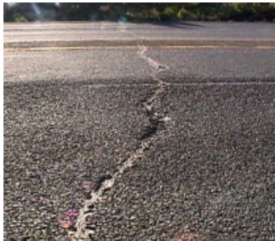
Figure 3.18: Thermal Cracking on US 97, ~MP 149, near Bend
