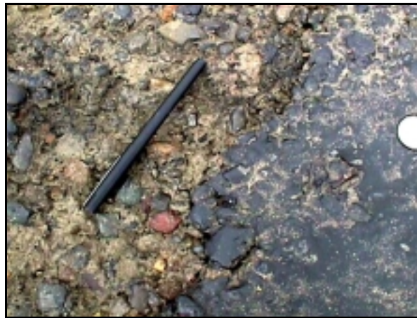
Figure 3.13: Close-up of Distress of Figure 3.12
