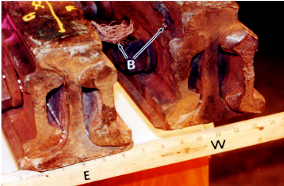
Figure 6. The accident joint bars. The east and west sections of the joint bars are indicated by "E" and "W." The location of the bond wires is indicated by "B." The bond wires are on the field side (outside) of the joint.
