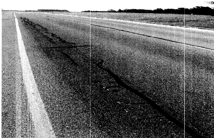
Figure 13. Structural Problems on SH 47.
