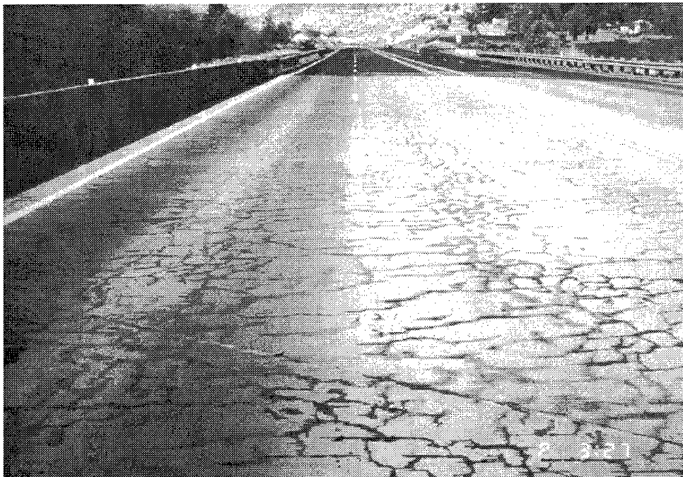
Figure 3.4: Sealed cracks in October 1995 distorted cracking severity.
