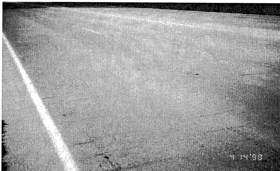
Figure 3.5: Typical transverse cracks (April 1998).
