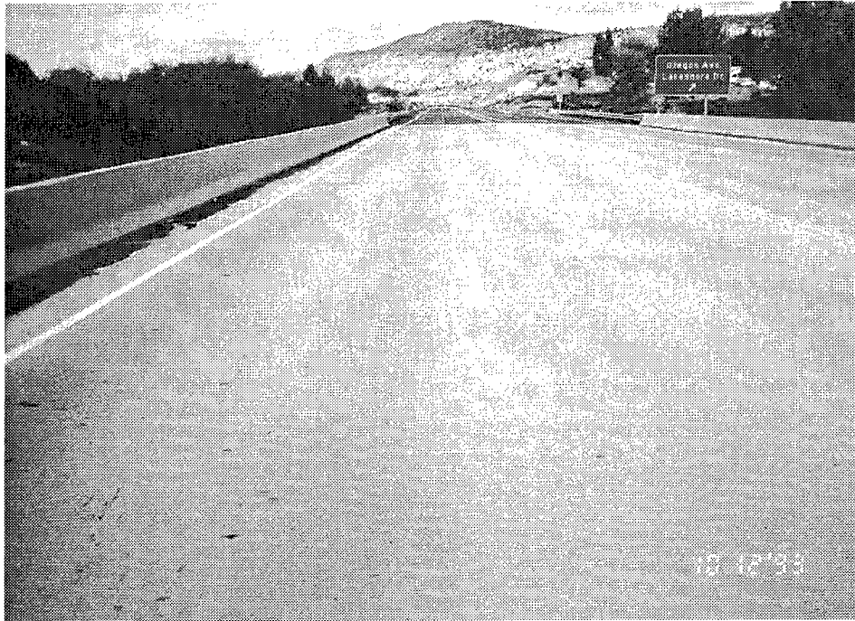
Figure 3.3: Transverse cracking was not visible (October 1993).
