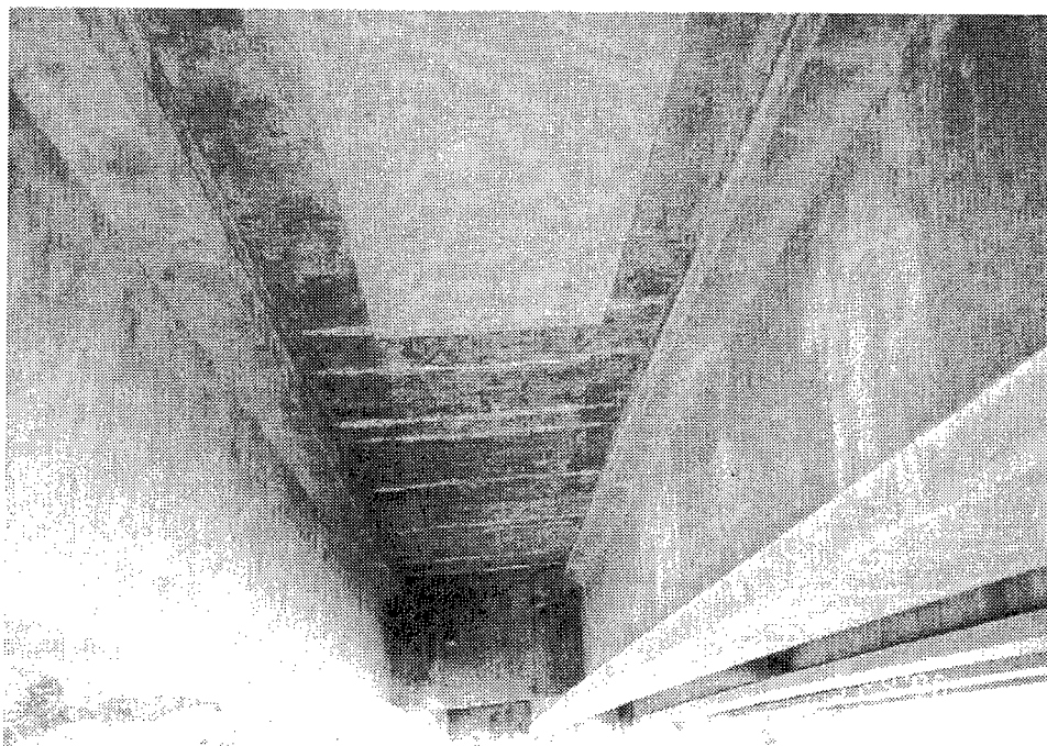
Figure 3.8: Transverse cracks were found on the bottom of the deck near center of span.
