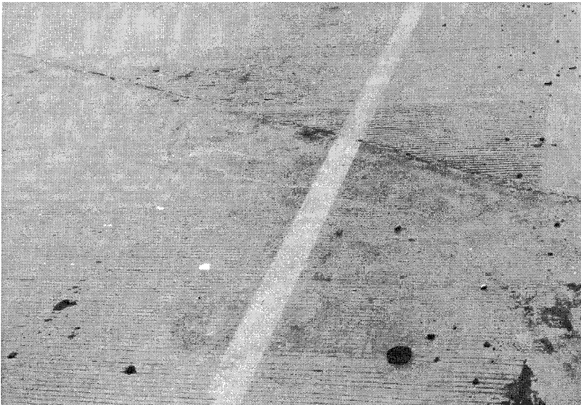
Figure 3.1: Cracks parallel to bents (April 1993).
