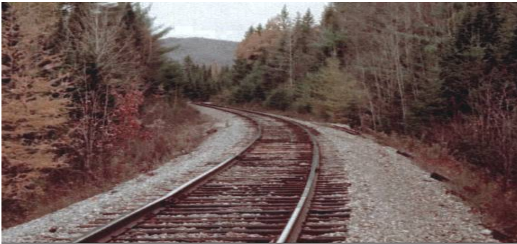
Figure 9: Typical “extensive treatment” track condition
