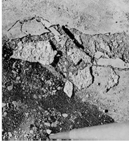
Figure 2.3 Scaling of concrete slab surface
