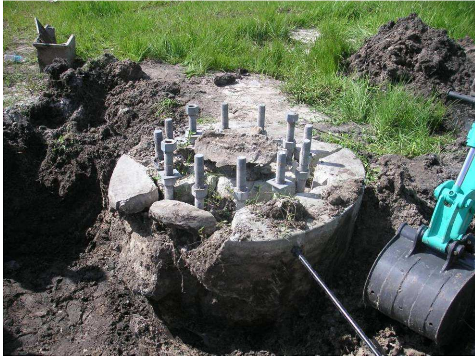
Figure 1-2. Failed foundation during post-failure excavation (1)
