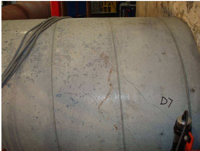
Figure 5-2. Formation of torsional cracks
