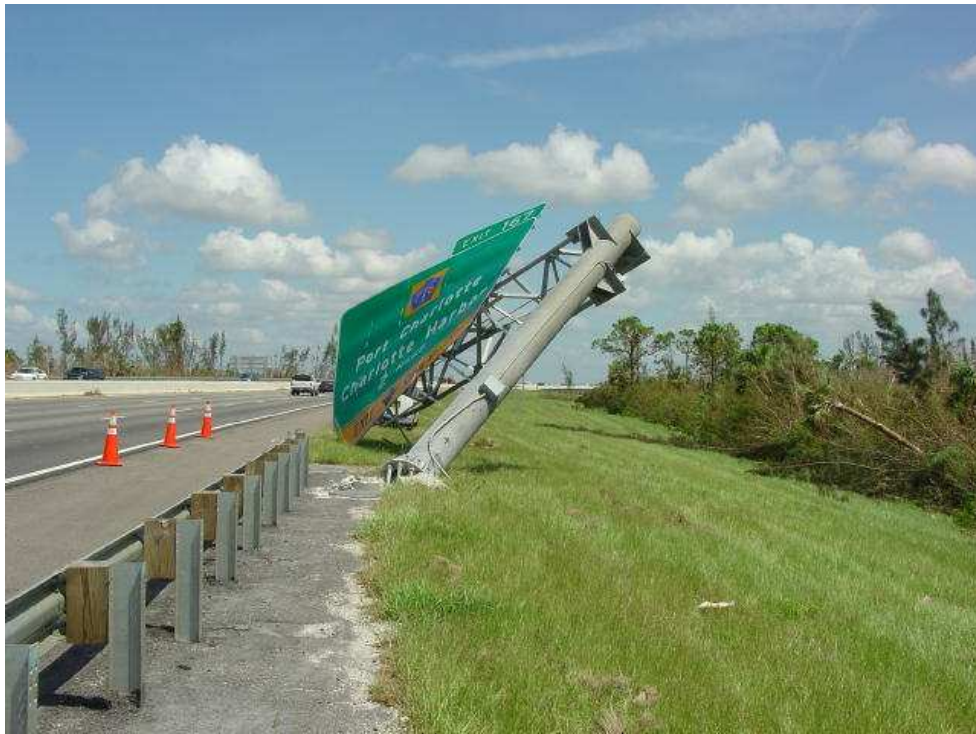
Figure 1-1. Failed cantilever sign structure (1)
