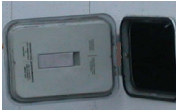
Figure 7-3. MCI Open Emergency Roof Exit Hatch – Exterior
