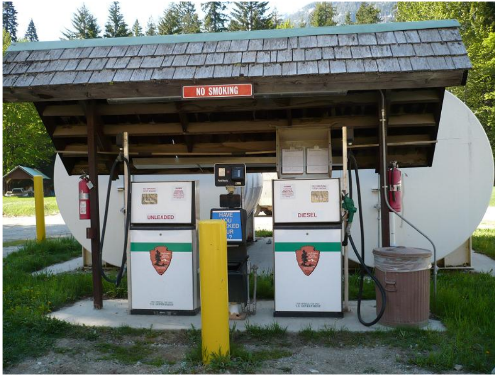
Figure 17 Fuel Storage and Dispensing Site at NOCA
