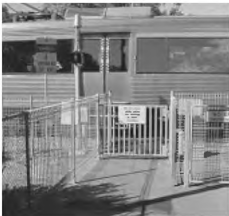
Crossing treatment on the suburban rail network in Perth. Gates automatically close when train is approaching. Users are alerted to the presence of approaching train by flashing lights and audible bells. Gates remain locked until trains have passed. Perth, Australia
