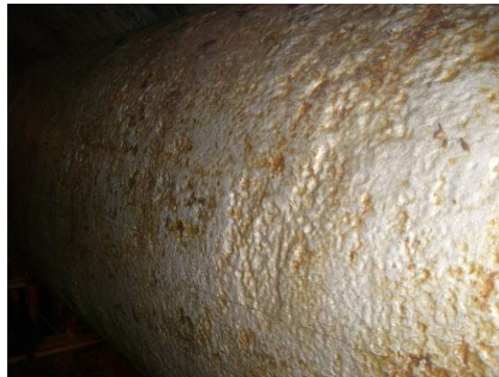
General corrosion located on much of the pipe
