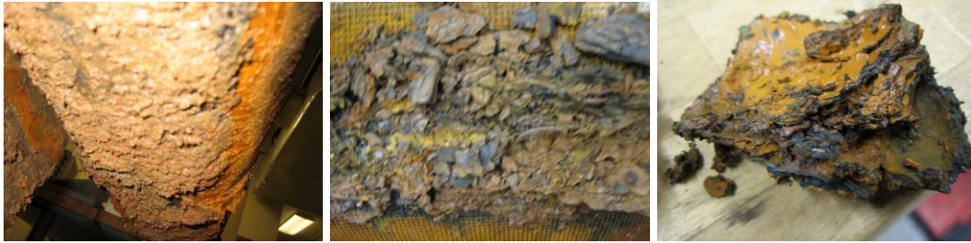
Figure 5. Corrosion products on the pipe surface
