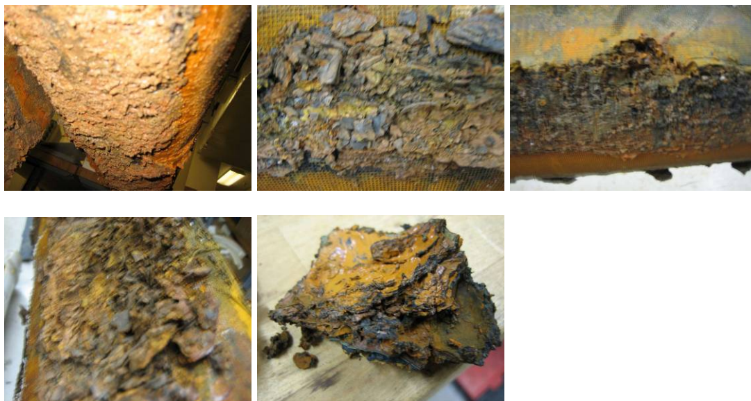
Figure 65. Photos of pipe surface on the bottom side (upper left), on sides (upper middle and right) and a piece of corrosion product (lower right)
