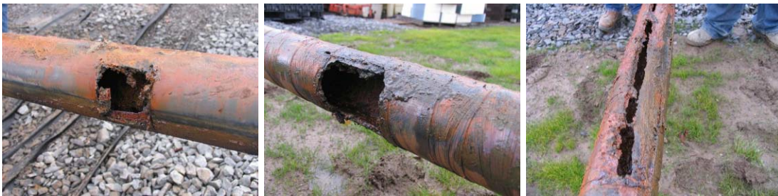
Figure 2. 1 st RG&E Test Pipe Defects: Large defects (left two) and 2.8% CSA defect at the weld location (right)
