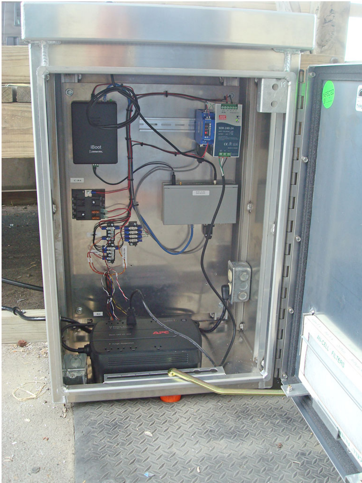
Exhibit 3. Representative Electronics Cabinet
