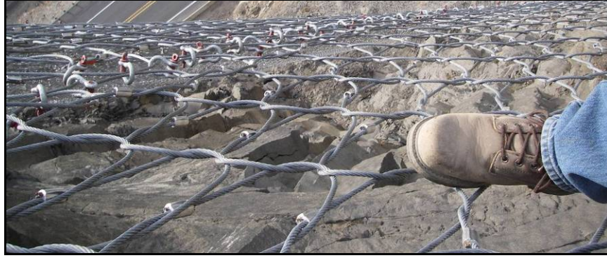
FIGURE 14. Deformation in upper portion of ROTEC ring nets.
