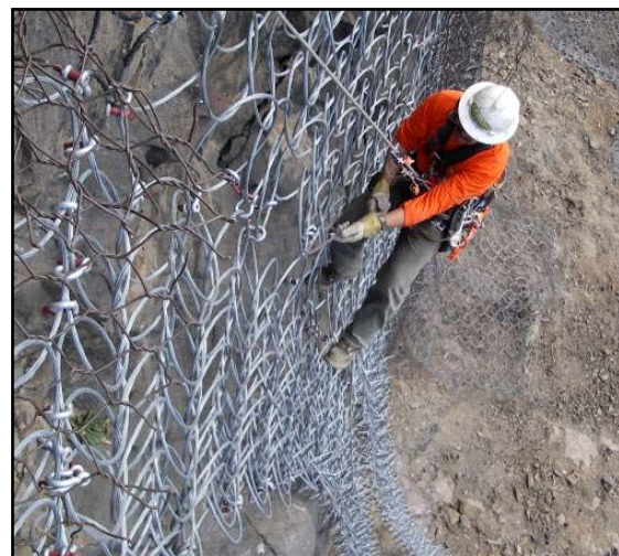
FIGURE 12. Seaming the contracted panels was extremely difficult, often requiring the use of a come-along to pull the seam together and secure the shackle.
