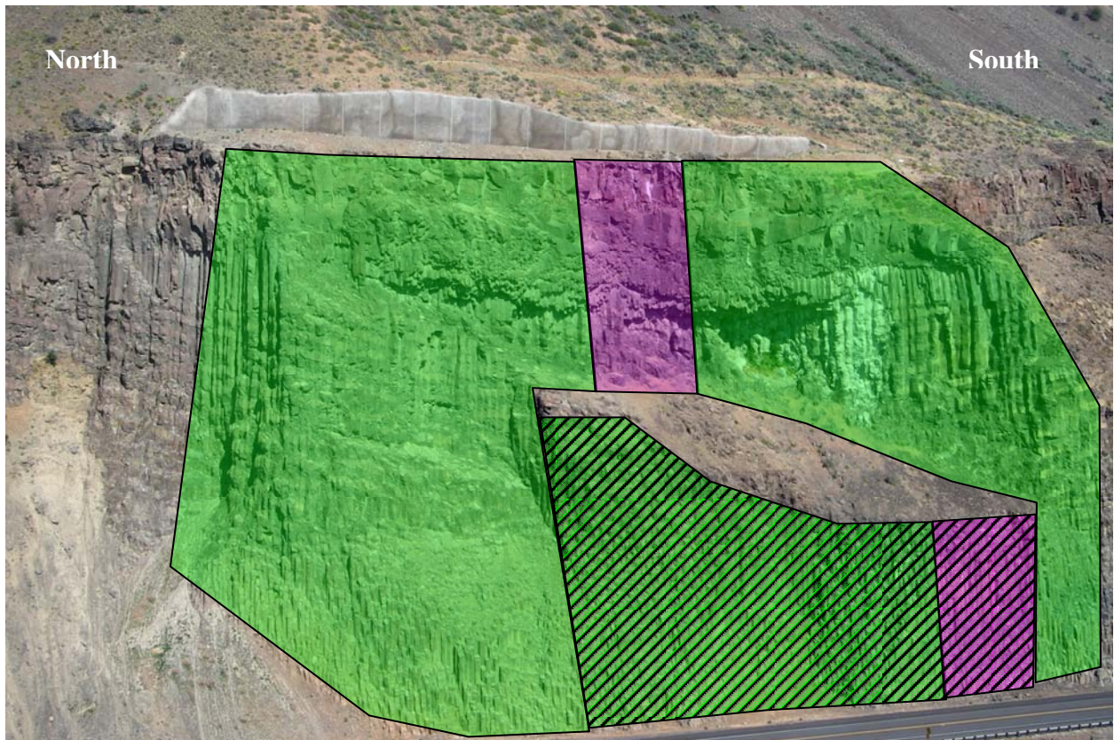
Figure 2. The green-shaded slope area depicts the ring net coverage, and the pink-shaded slope area would be the control sections of cable net coverage. The fabric coverage areas that extend to the slope crest would be a standard application secured by a top horizontal rope and series of anchors located above the slope crest. The diagonal-lined portion represents the modified installation that would be exposed to sub-horizontal impacts from rocks exiting the upper standard drapery.
