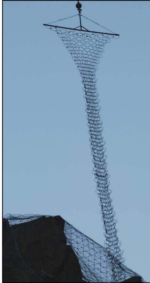
FIGURE 10. Maccaferri ring net with wire mesh backing exhibited severe contraction within the panels.
