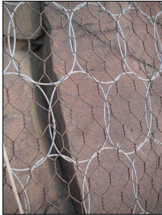
FIGURE 9. Slight elongation noted in IGOR rings where panels were heavily loaded.
