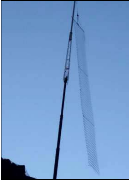
FIGURE 8. IGOR ring net panels without wire mesh maintained their rectangular shape when lifted.
