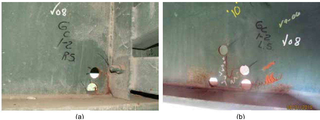
Figure 3.2: Cracking at the Instrumentation Location on the (a) Stiffener Side (b) Non-Stiffener Side
