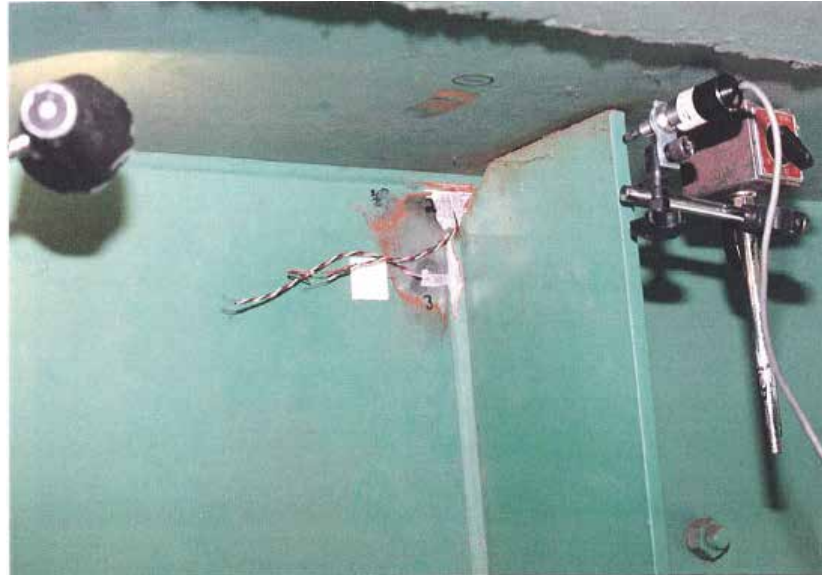
Figure 3.5: Photograph of LVDT Placement Similar to that Used in the First and Second Field Test
