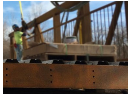
Weathering steel has a rusty surface that protects the steel from environmental damage.
