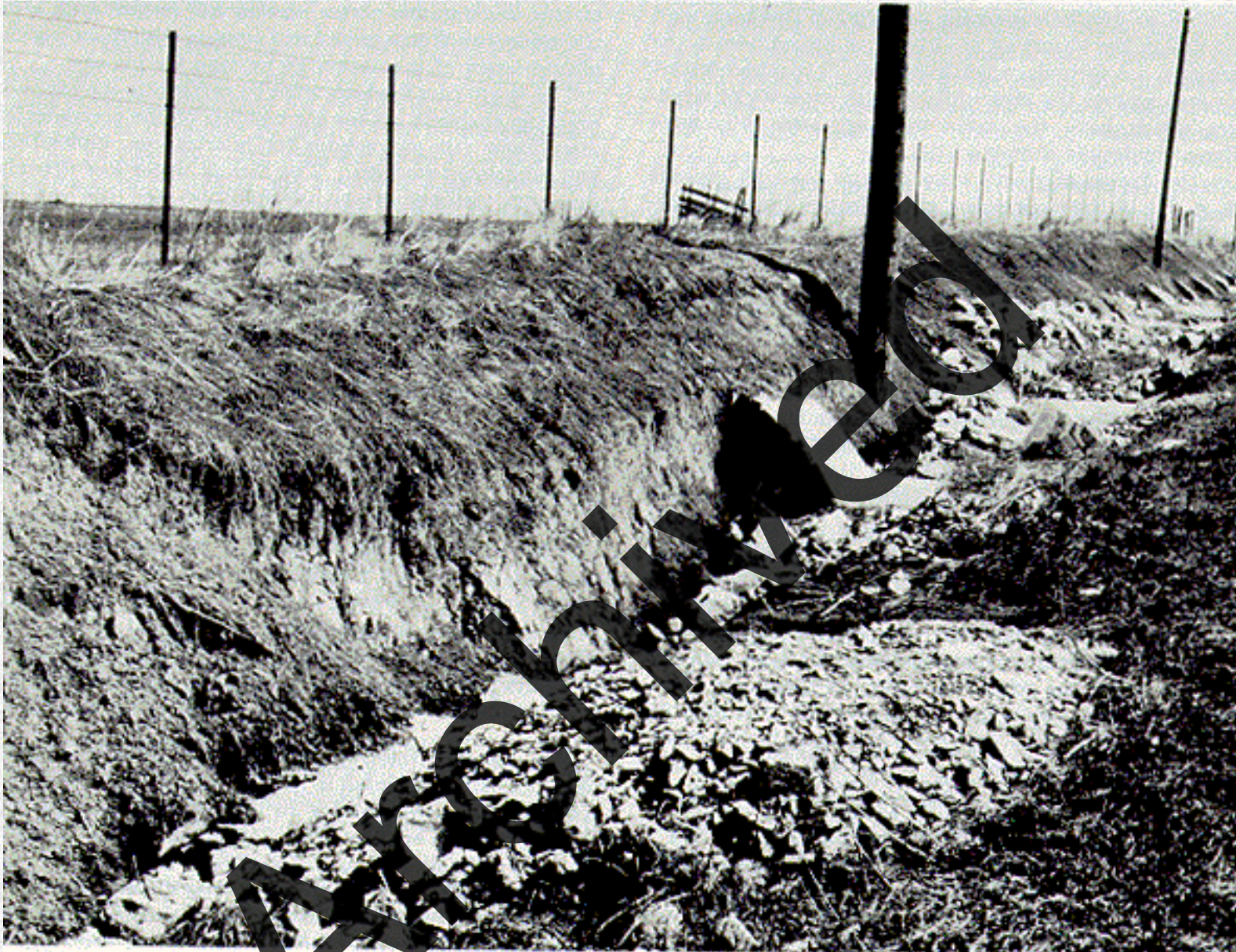
Figure 4. Poorly Designed Ditch Checks
