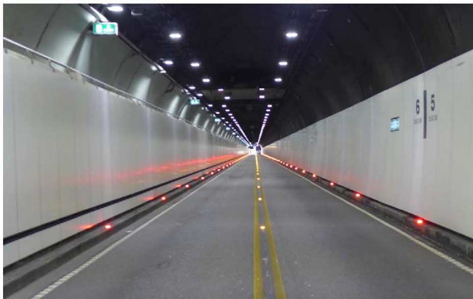
Figure 2-65: Mount Victoria Tunnel roadway marking lighting demonstration.
