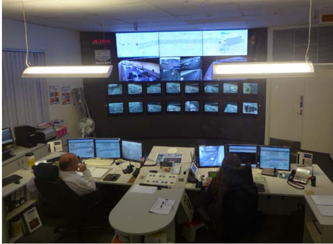
Figure 2-37: Sydney Harbor Tunnel control room.
