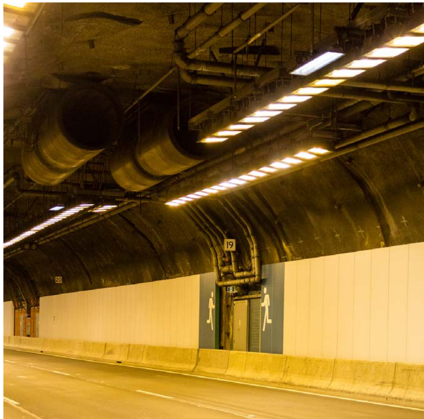
Figure 2-62: M2 Tunnel emergency exit signage.
