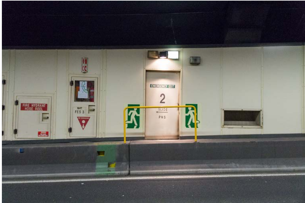
Figure 2-61: Sydney Harbor Tunnel emergency exit signage.
