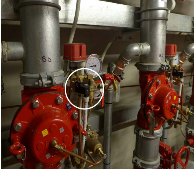
Figure 2-31: Waterview Tunnel FFFS valve regulator.
