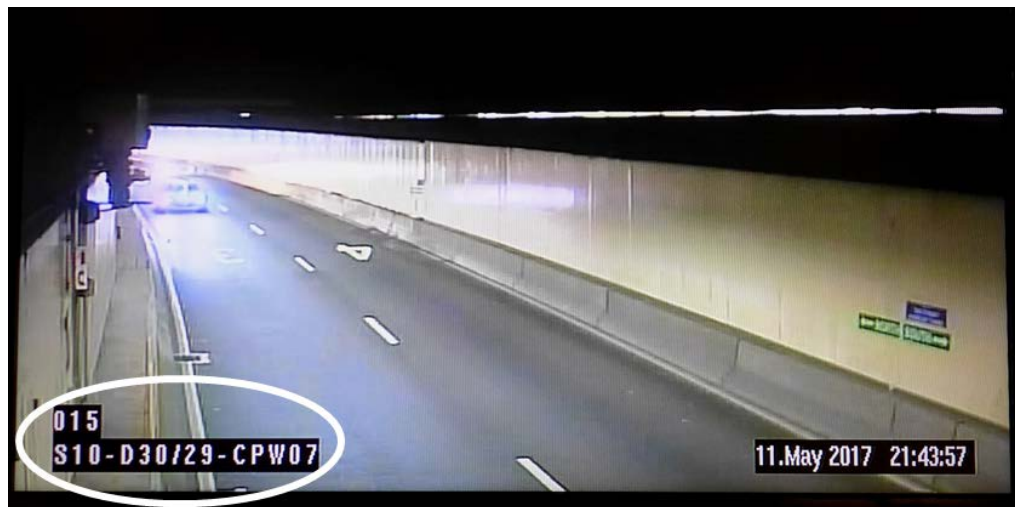
SOUTHBOUND TUNNEL DELUGE ZONES 30/29 CROSS PASSAGE 7
