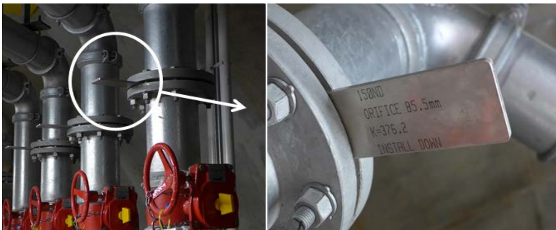
Figure 2-30: Waterview Tunnel FFFS valve with orifice plate.
