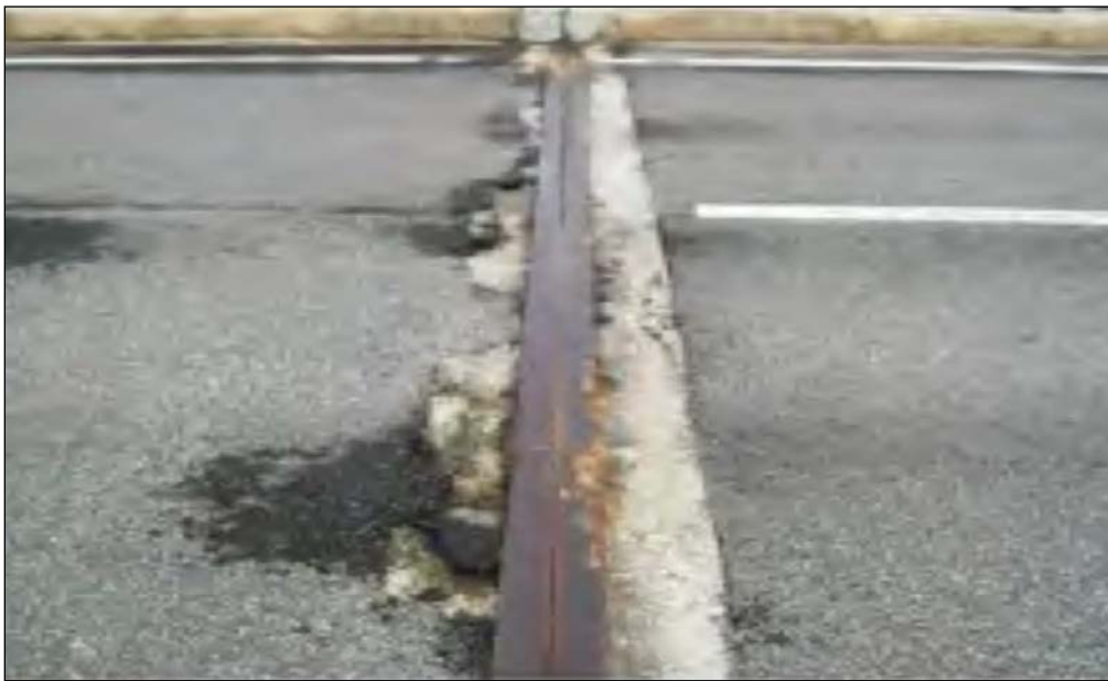
Figure 11. Failed deck joint condition.
