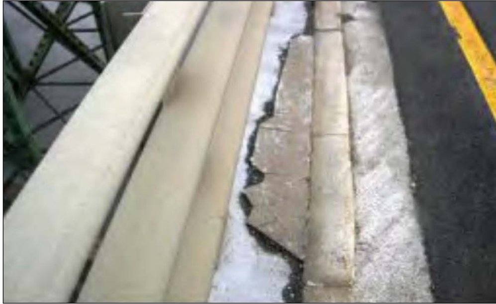
Figure 12. Salt-laden runoff at curb.
