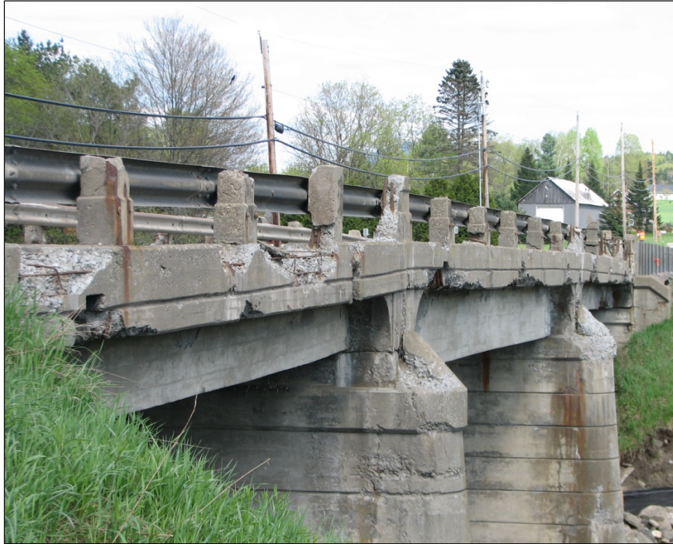
Figure 2. The functionally obsolete existing structure.
