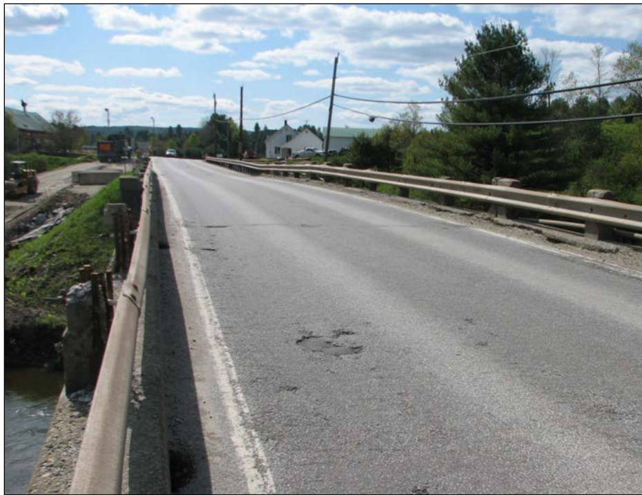
Figure 3. Deteriorated bridge deck.
