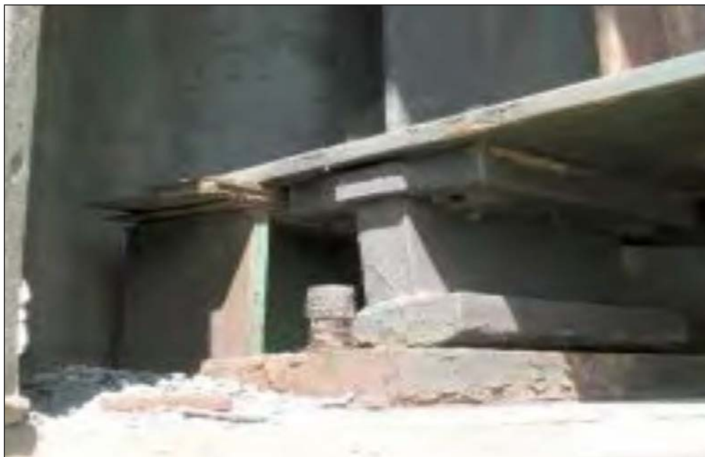
Figure 13. Corroded bearing condition.
