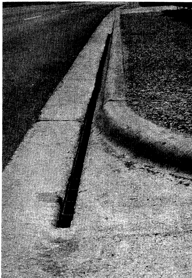
Figure 18. Slotted drain inlet at an intersection.
