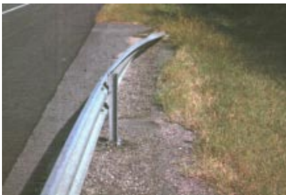
Figure 13. Breakaway cable terminal (BCT).
