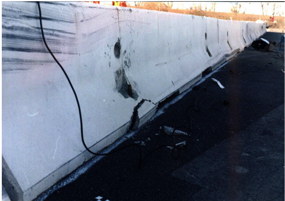
Figure 2-15 - Backside of Barrier Post Impact
