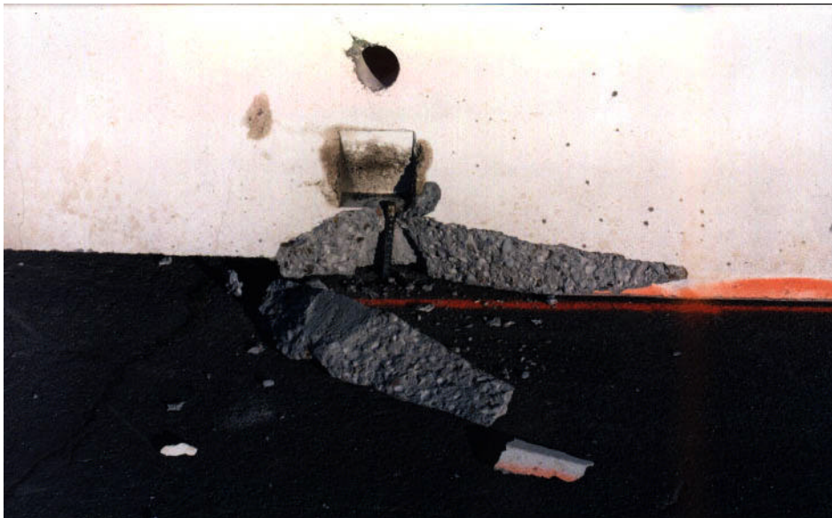
Figure 2-12 - Concrete Spalling At Anchor Stake
