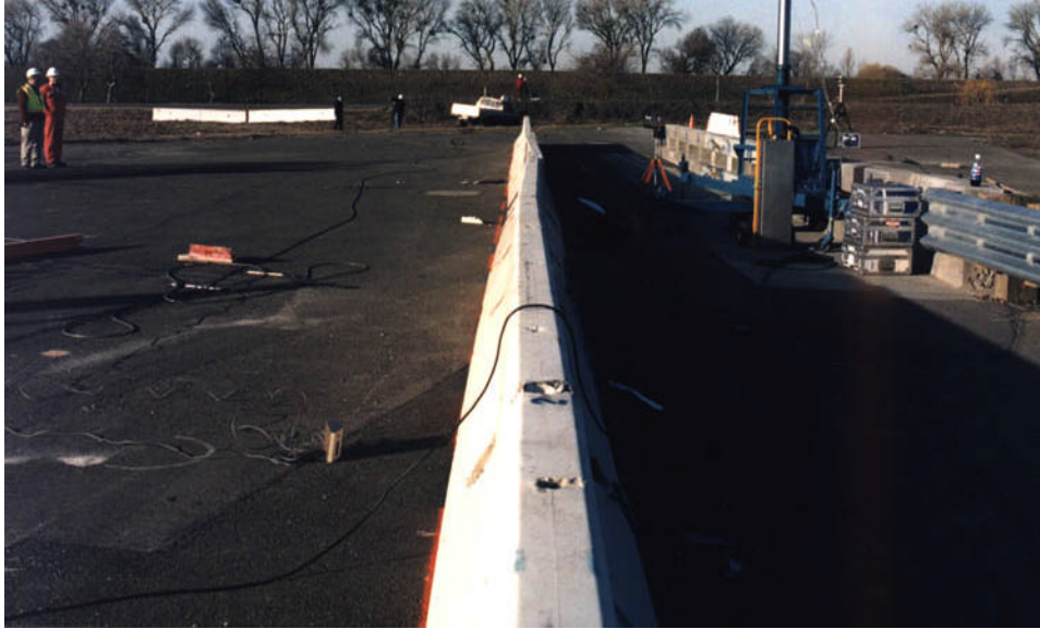
Figure 2-14 - Downstream View of Barrier Post Impact
