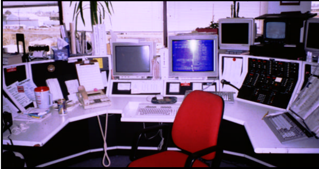
Figure 6. CAD/AVL and Legacy VAX Equipment at a Dispatcher's Console
